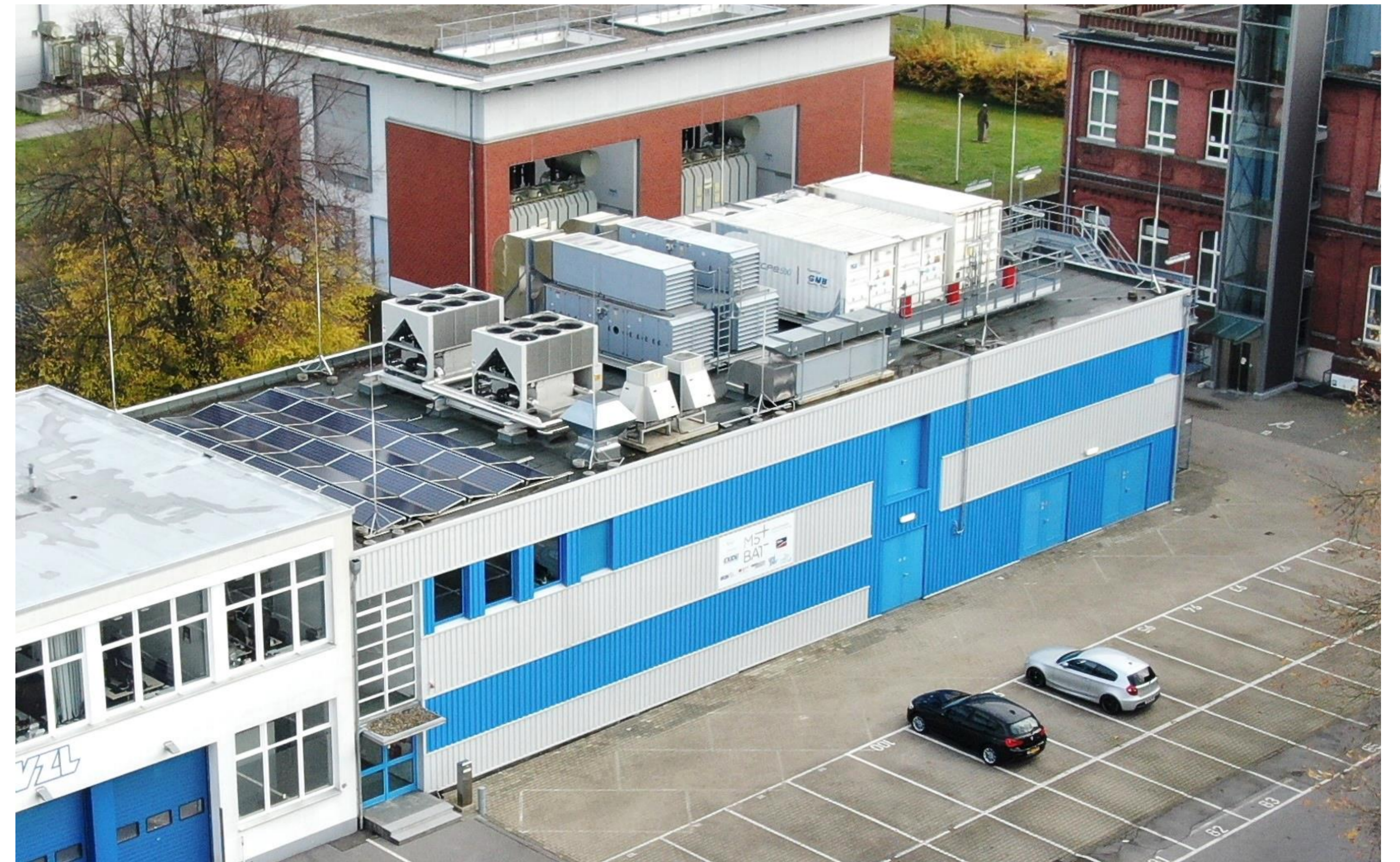
Figure 1: Battery storage M5BAT, Aachen, Hüttenstraße 9
